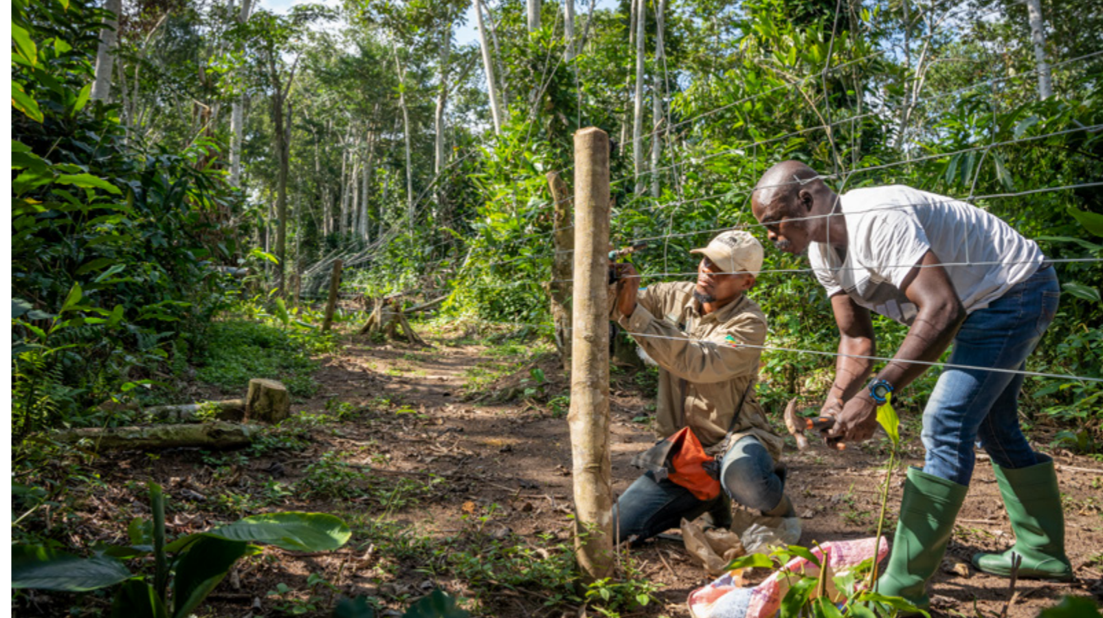
Above: In Odzala-Kokoua National Park, Congo, a 20 km solar-powered elephant-proof fence has proven highly effective in safeguarding crops of local farmers © Irene Galera
